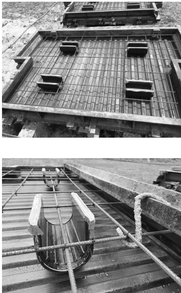
Fig 3.3: The complete assemblage of reinforcement and SC connectors with opening sealed with tapes
